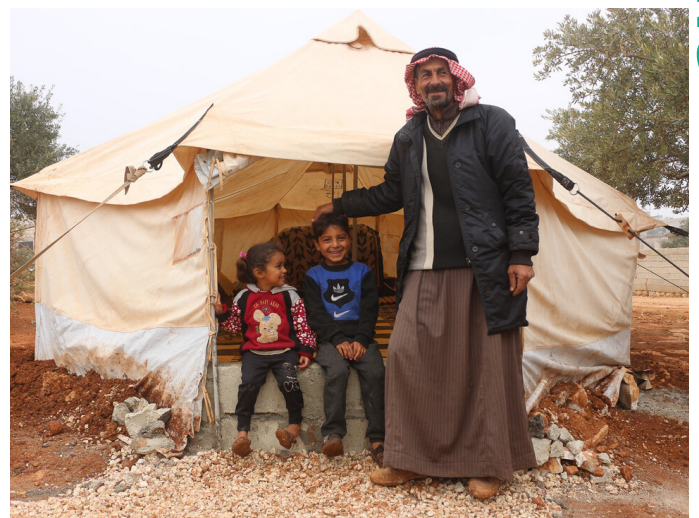
Abu and his two children were one of the 800 families to receive tent levelling support - a concrete base, raising their tent off the ground.
